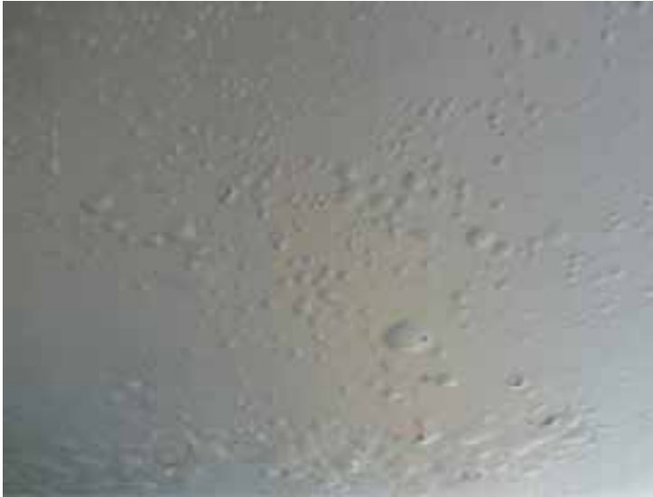
Osmoseschaden in fortgeschrittenem Stadium
